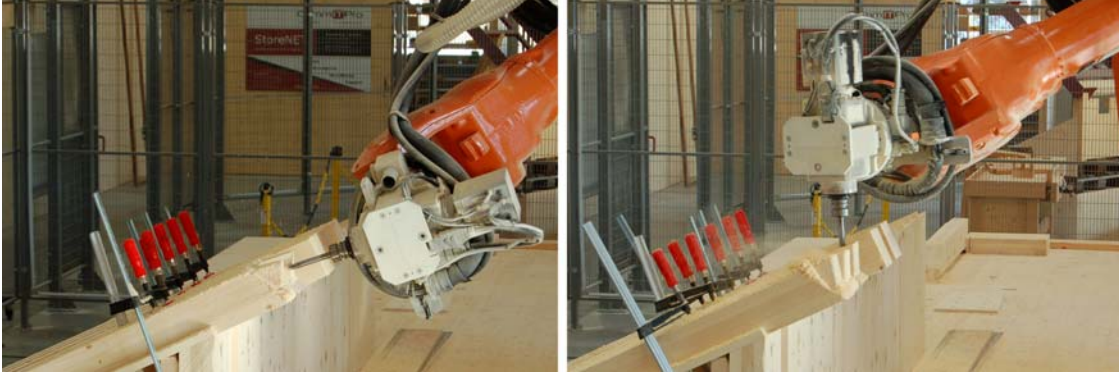
Figure 8 Positioned wooden beams and robot milling head during the production of the two different joint parts.
